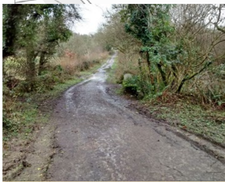
Upgrade to smoother surface and repair potholes. Upgrade to sealed surface to protect bridge structure?
