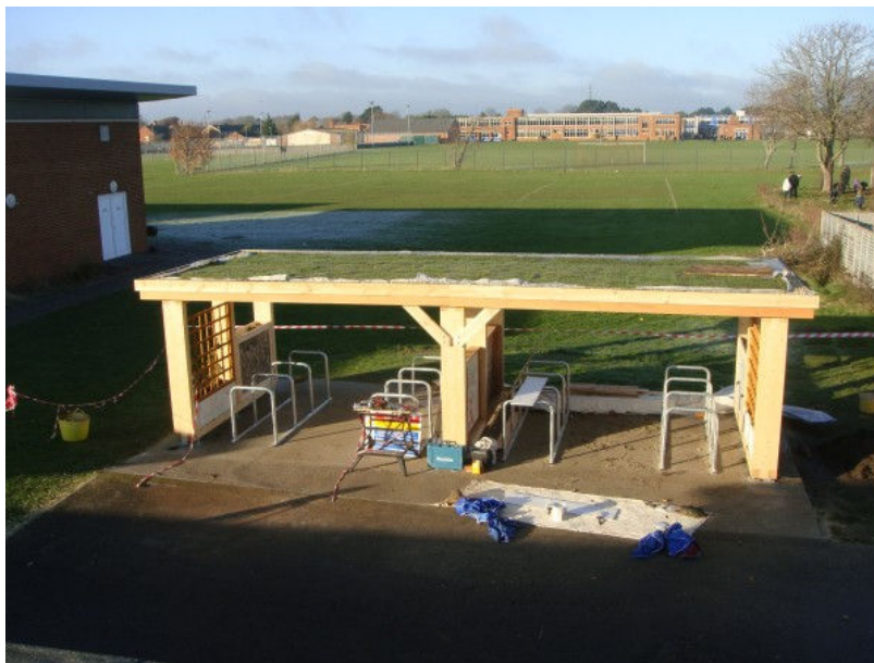
The new shelter just prior to completion, with view of the green roof
