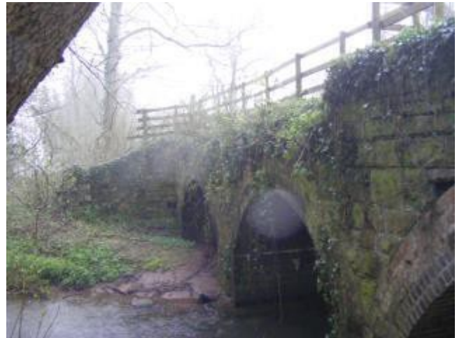
Figure 9. Bridge over Berthin Brook, with some bat features and likely use by otters
