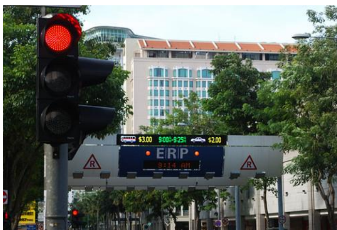
Singapore ERP charging gantry, Creative Commons Image
