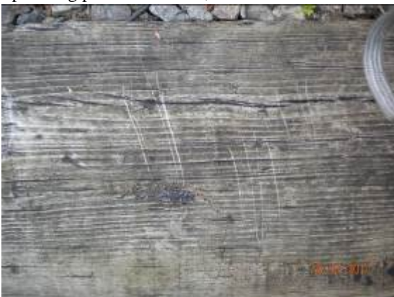
Scratch marks, track sleeper
