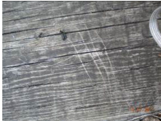
Scratch marks, track sleeper
