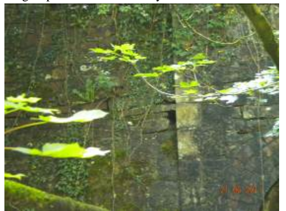
Cracks in wall of overbridge, Brynmenyn colliery
