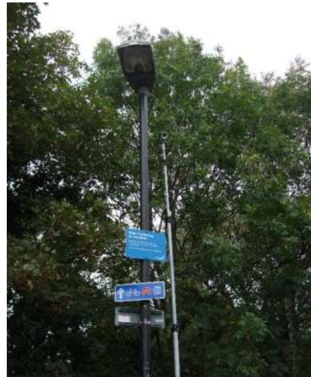
Image: Video monitoring equipment at Site Two
